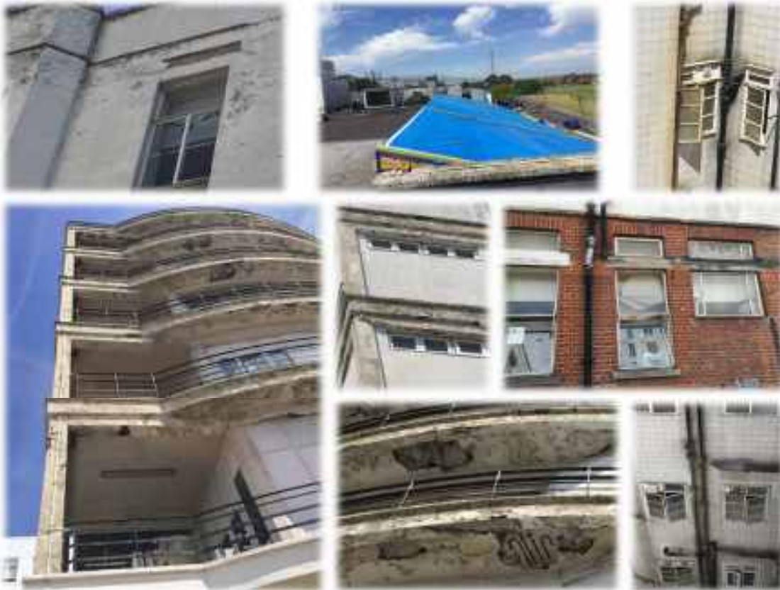
Figure 5: Examples of quality of St Helier Hospital buildings
