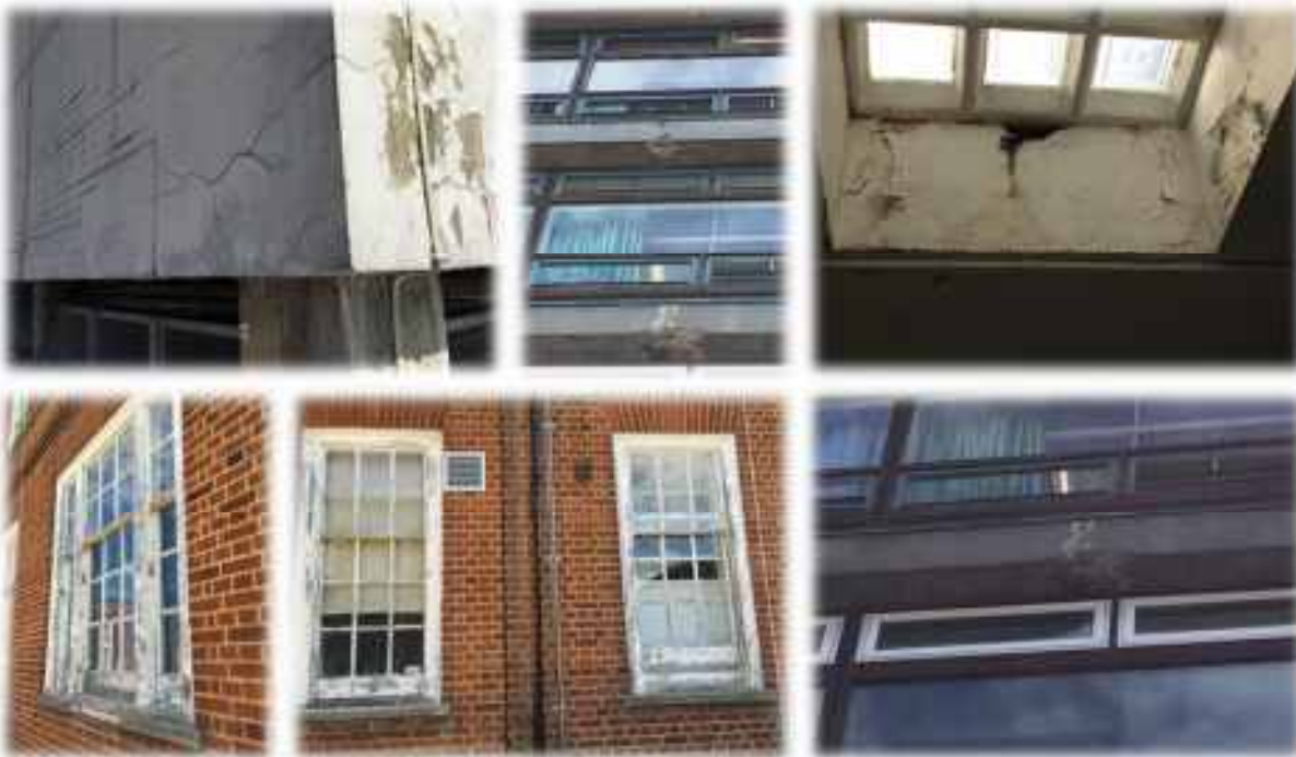
Figure 3: Examples of quality of Epsom Hospital buildings
